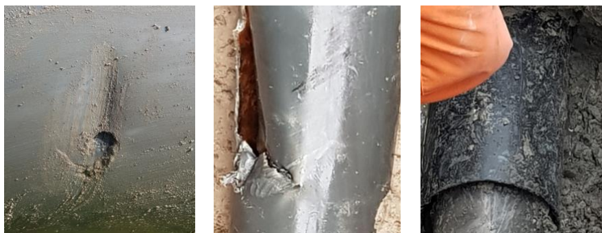
Figure 2. In-situ footage after excavation of Pipe 4 (left) and Pipe 5 (middle) with break due to 3 rd party impact, and Pipe 7 (right) with crack due to poor installation quality.
