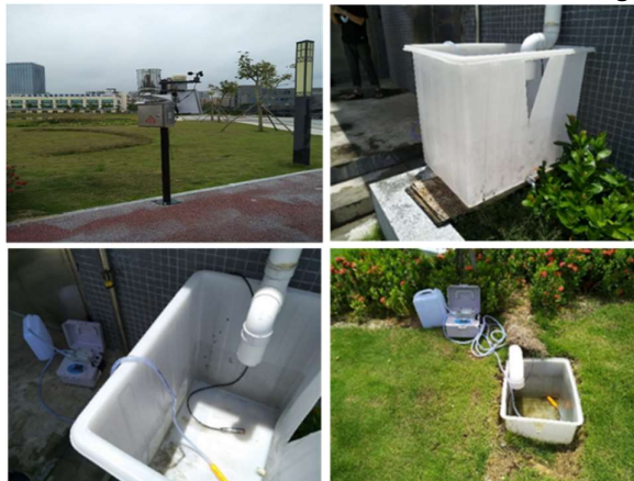
Figure 3 Flow monitors and weather station installed at the site.
